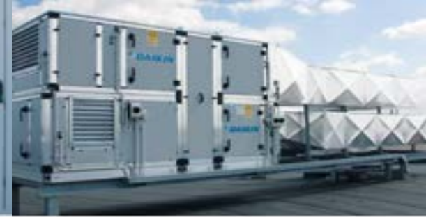
Air handling units
